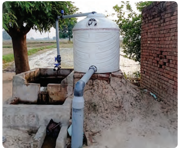
Water Holding Tank at an Average Height of 1m
